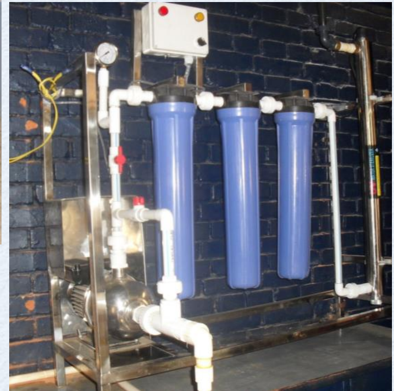
Water purification in SSP Canteen
